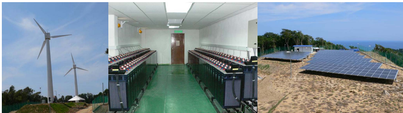
Figure 10: Lead-acid battery installation in a 500 kW renewable sources power plant with combined eolic and photovoltaic generation
