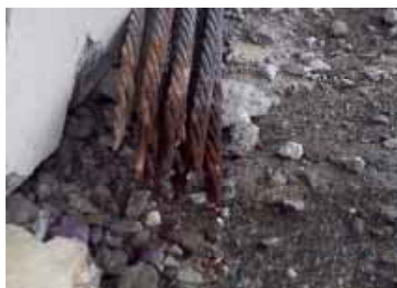
Figure A.1.7: Photo from broken tendon cables
