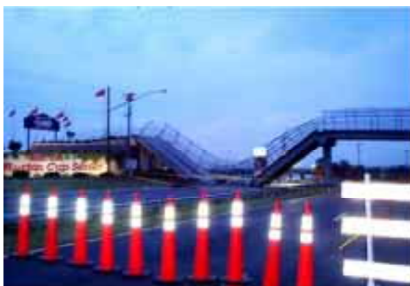
Figure A.1.6: Photo from a bridge collapse (cause: broken tendon cables) [5]
