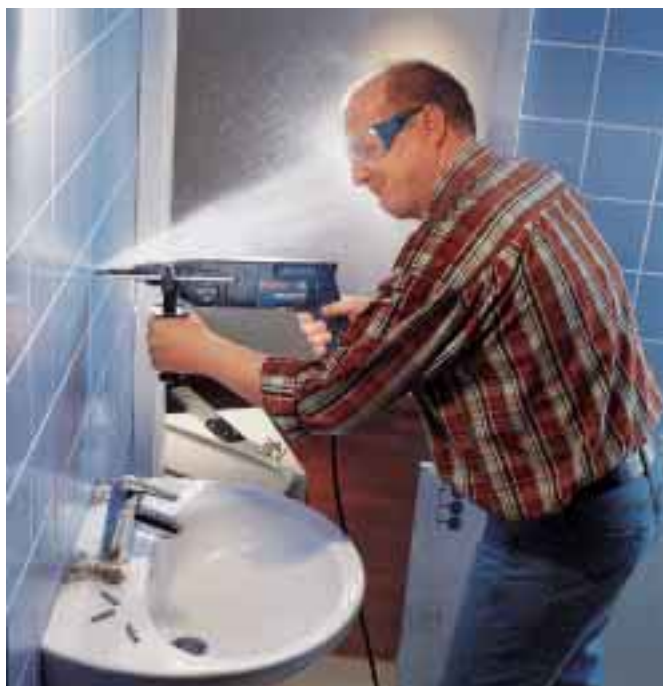
Figure A.1.3: Scenario for drilling into a plastic water pipe without the use of such a UWB sensor device
