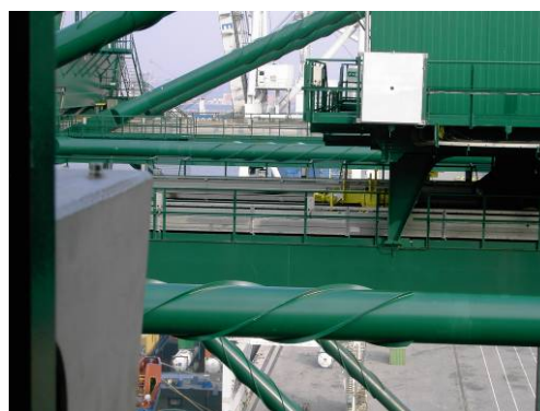
Figure A.4.1.4: STS, RTG, RMG cranes
